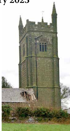
The church tower with its missing pinnacle following the lightning strike in 2012.
