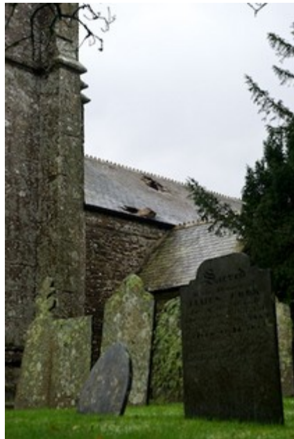
Holes in roof over the entrance porch
