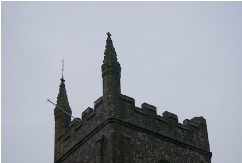
Flag pole leaning askew
