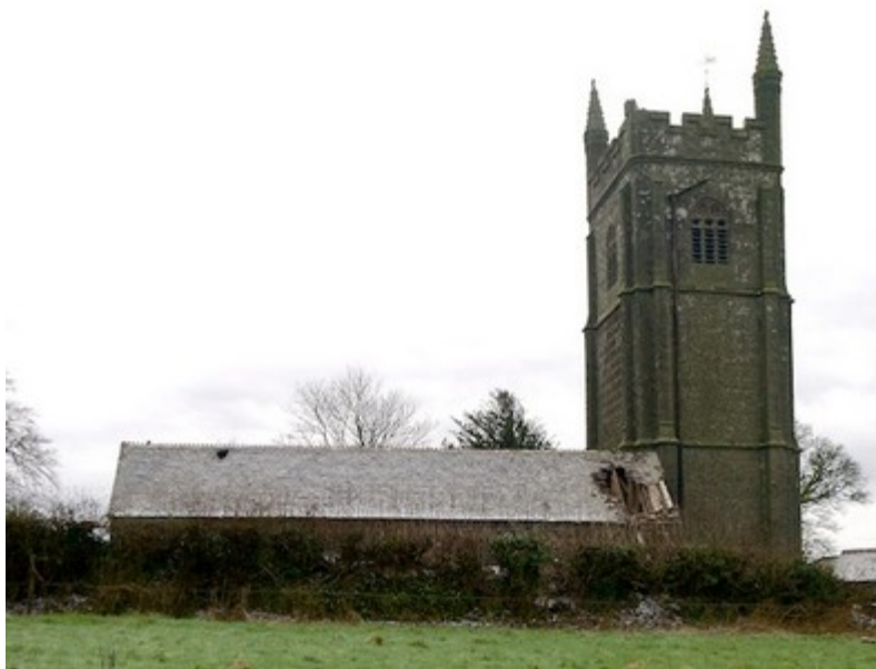
Showing holes in roof and gap on the tower
