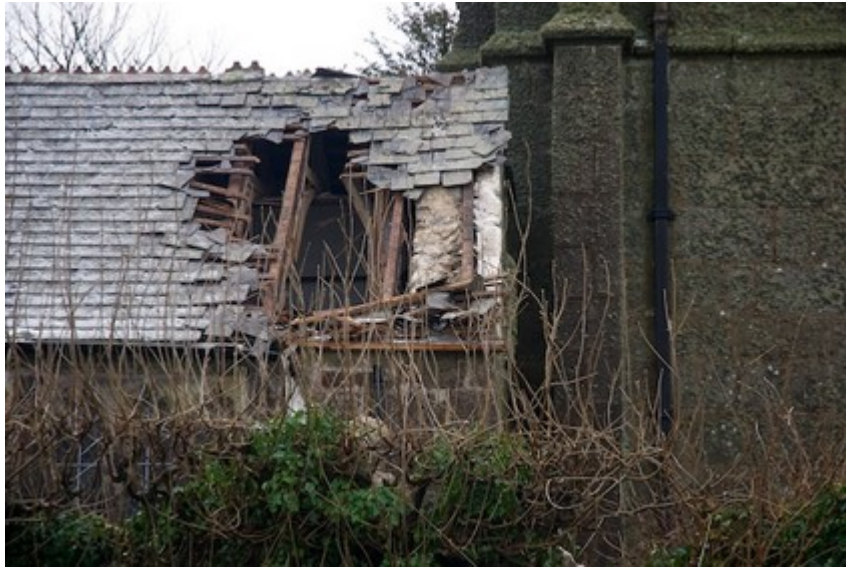
Hole in the roof of the north aisle
